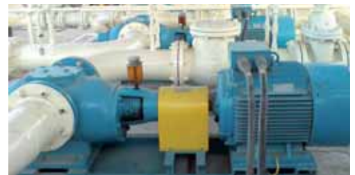
2 Leistritz HFO Unloading Pump L2NG
